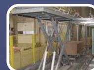
Automatic transport systems
